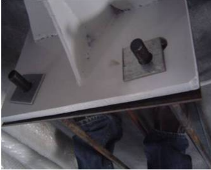
Lift the pole with a crane and put it on the foundation.
